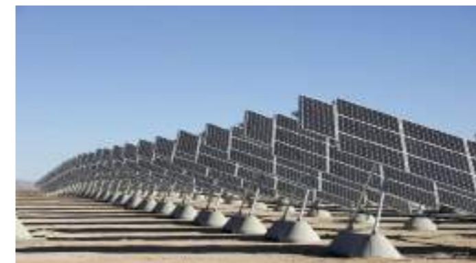
Utility-Scale Solar + Storage (3MWh)
