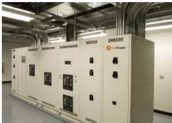
Indoor Data Center Power Pack System
